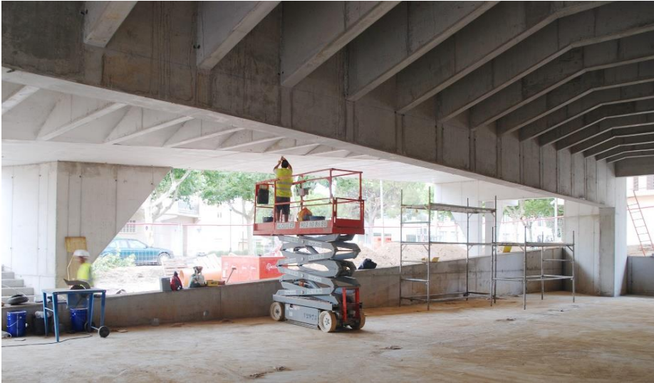
Figure 5: Concrete beams of the new hall supporting the new square (the roof of the hall).
